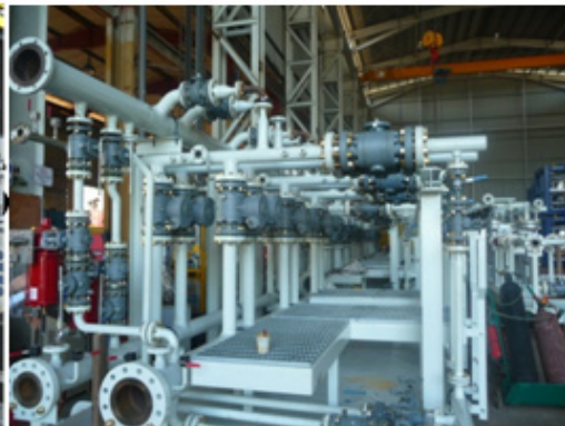
PLATFORM PRODUCTION MANIFOLD
